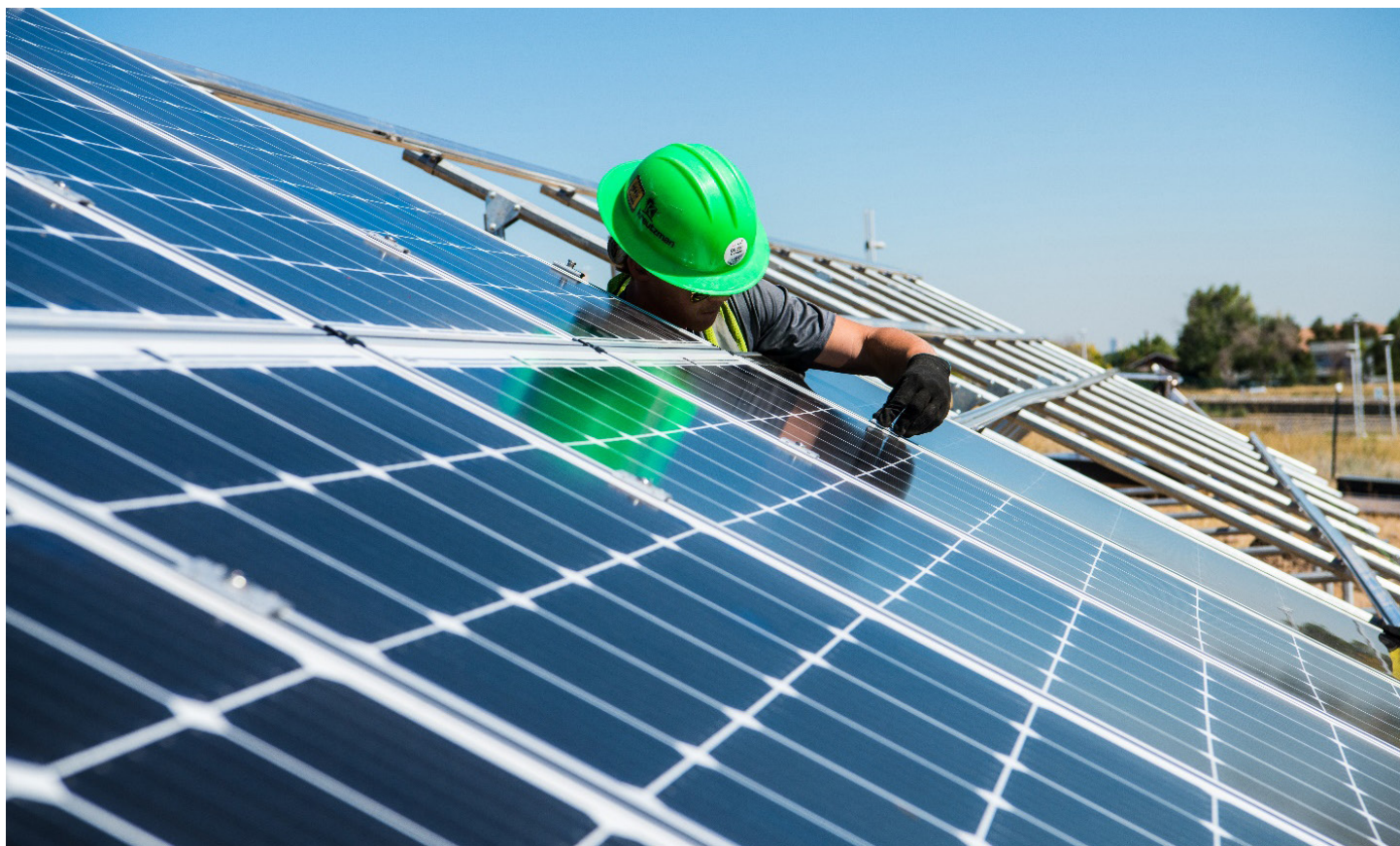
A worker with Zilla Rack installing photovoltaic modules on a rack of solar panels just north of the National Renewable Energy Laboratory (NREL) parking garage in Golden, Colorado, on September 28, 2016.
