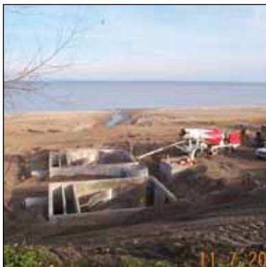
(a) Installation of a system for removal of solids from stormwater. The photo was taken in late 2000.
