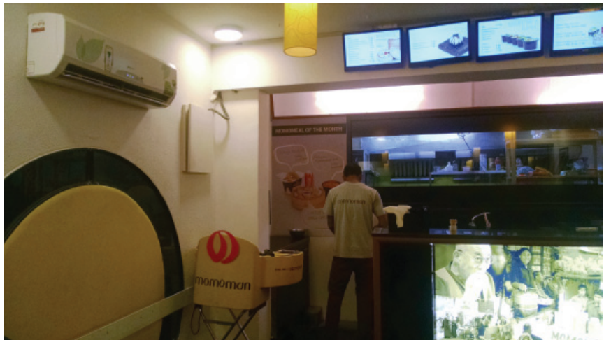
Hydrocarbon AC in use at a commercial establishment in Gujarat
