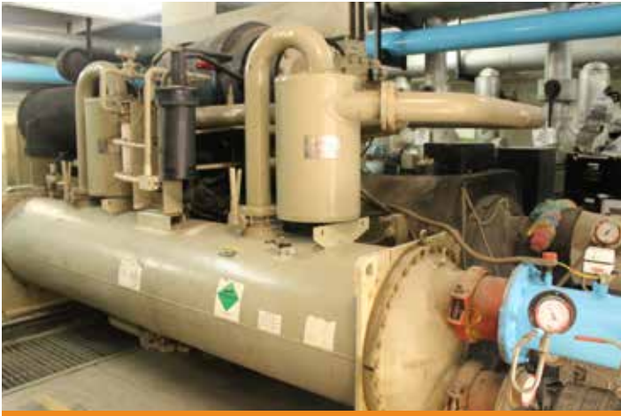
RETROFITTED CHILLER SYSTEM, MAHINDRA TOWERS.
