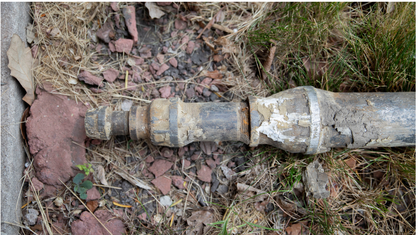
A close-up view of part of a lead service line removed from outside a home.
