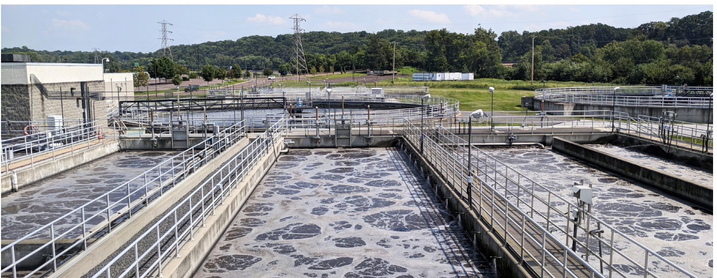
Water in an aeration tank at Oaks Wastewater Treatment Plant in Pennsylvania.
