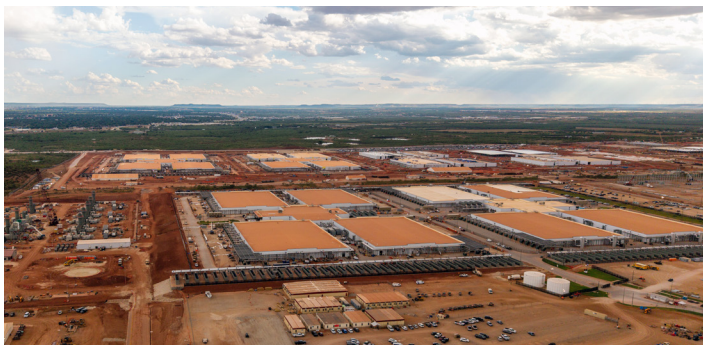
The Stargate AI data center under construction in Abilene, Texas, on September 23, 2025
