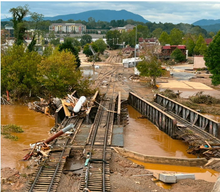
A damaged railroad bridge in Asheville, North Carolina, following flooding on the Swannanoa River during Hurricane Helene.
