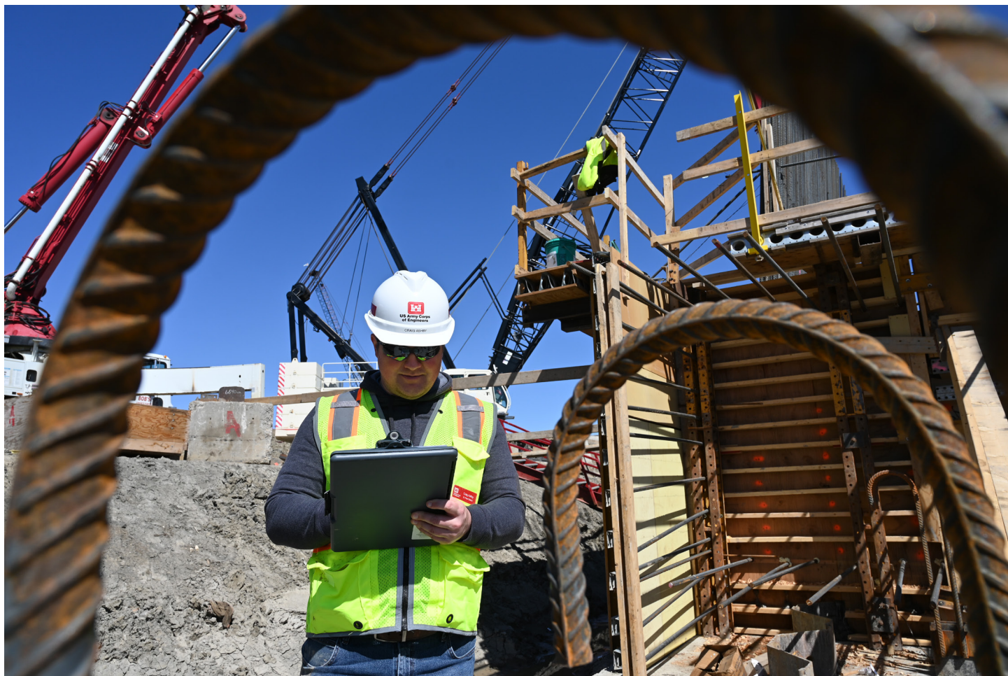
An engineer monitors construction of the Red River Structure, a major component of the Fargo-Moorhead Metropolitan Flood Risk Management Project.
