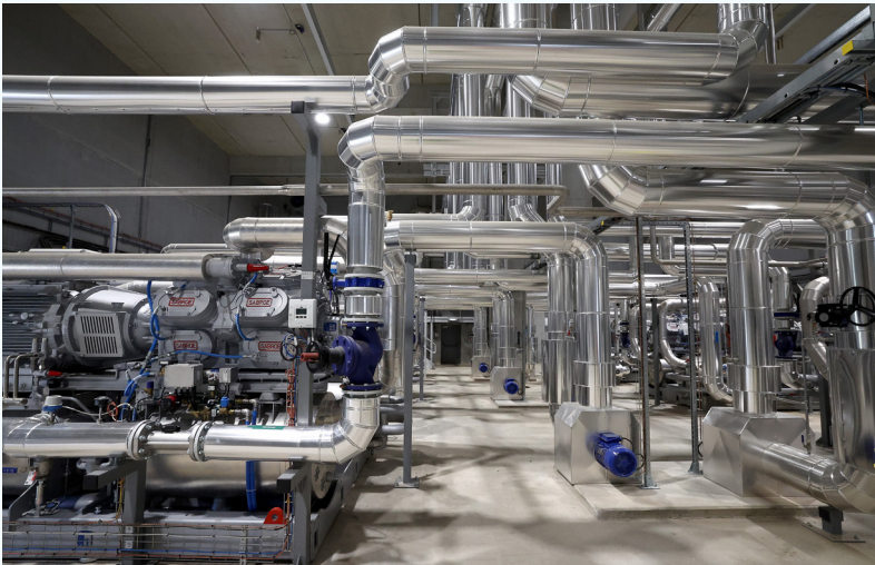
An industrial heat pump at the EVOS project of the Strasbourg-West district heating network in Strasbourg, France, on July 17, 2025.
