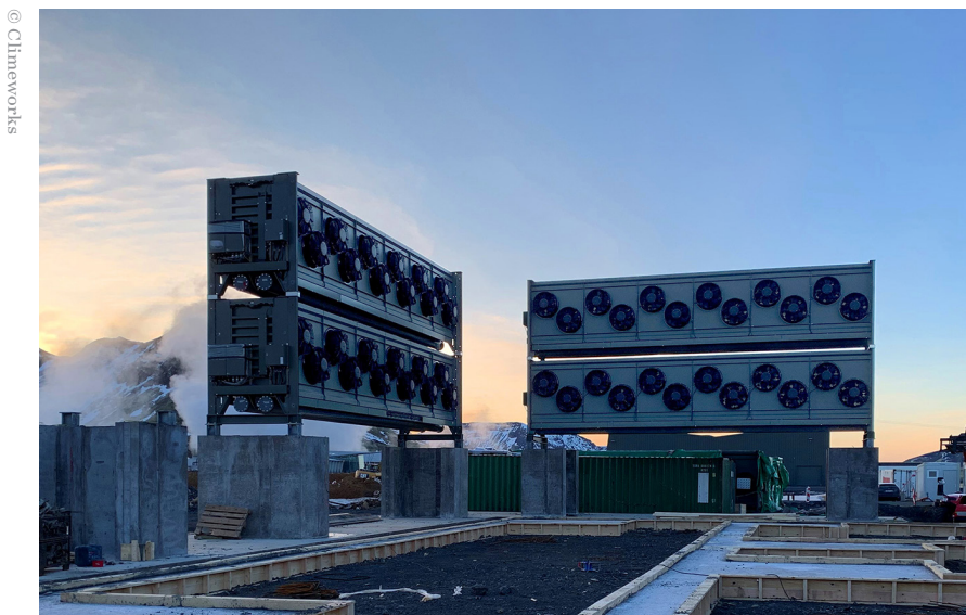
Fans pulling in large volumes of ambient air at Climeworks' Orca direct air capture plant (a form of CDR) in Iceland.
