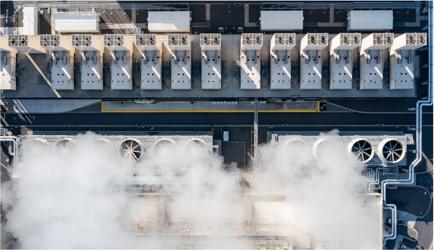
Industrial cooling systems on a rooftop at the Dalles Google Data Center, a hyperscale data center in the Dalles, Oregon.
