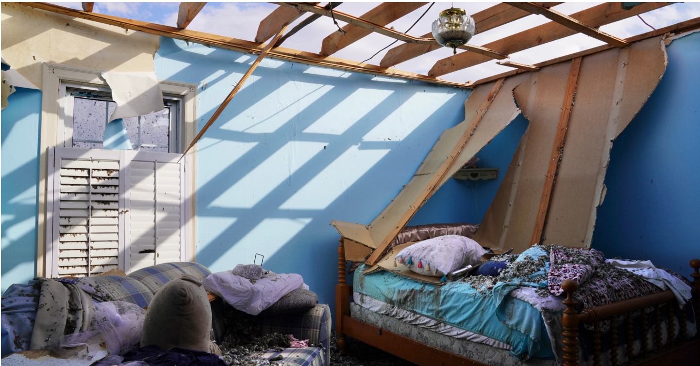
Roof damage caused by strong winds can lead to cascading and devastating impacts for homes and the families that reside in them. For insurers, roof-related damage results in 70-90 percent of all catastrophe-related insurance losses in most years.
