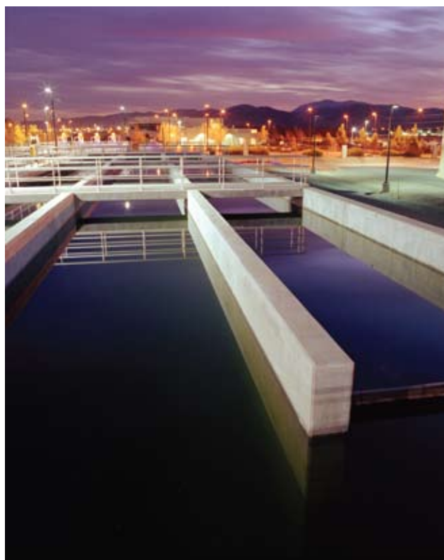
Wastewater recycling facility at Delta Diablo.
