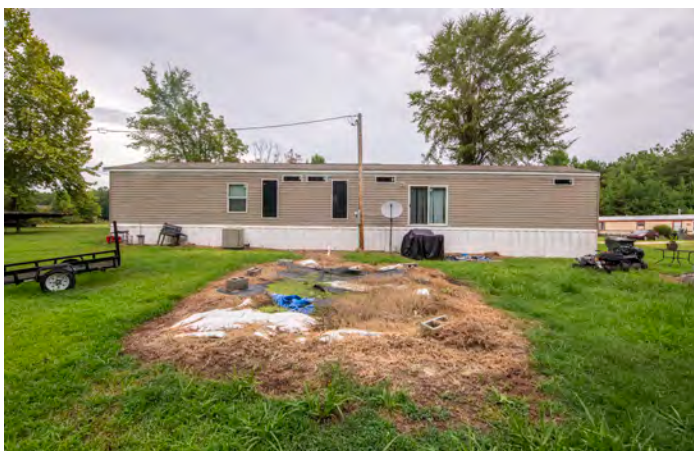
A home with a failing septic system resulting in a surface pool of sewage in Hayneville, Lowndes County, Alabama, on August 1, 2022.
