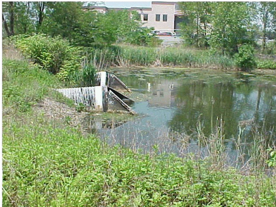
Photo 2: View north of the twin outlet structures. Note the inlets to the outlet pipes have separated at the joints.
