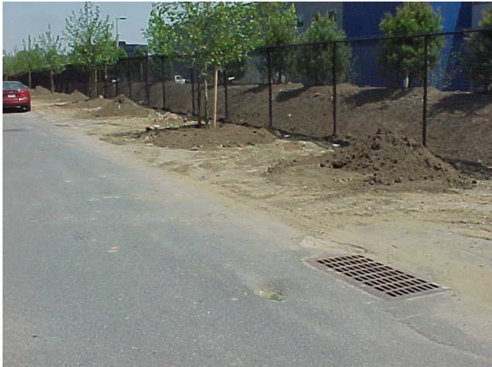
Photo 1: View west of construction along 15th Avenue. Note no BMPs along site fence and soil had entered the avenue by three inlets.
