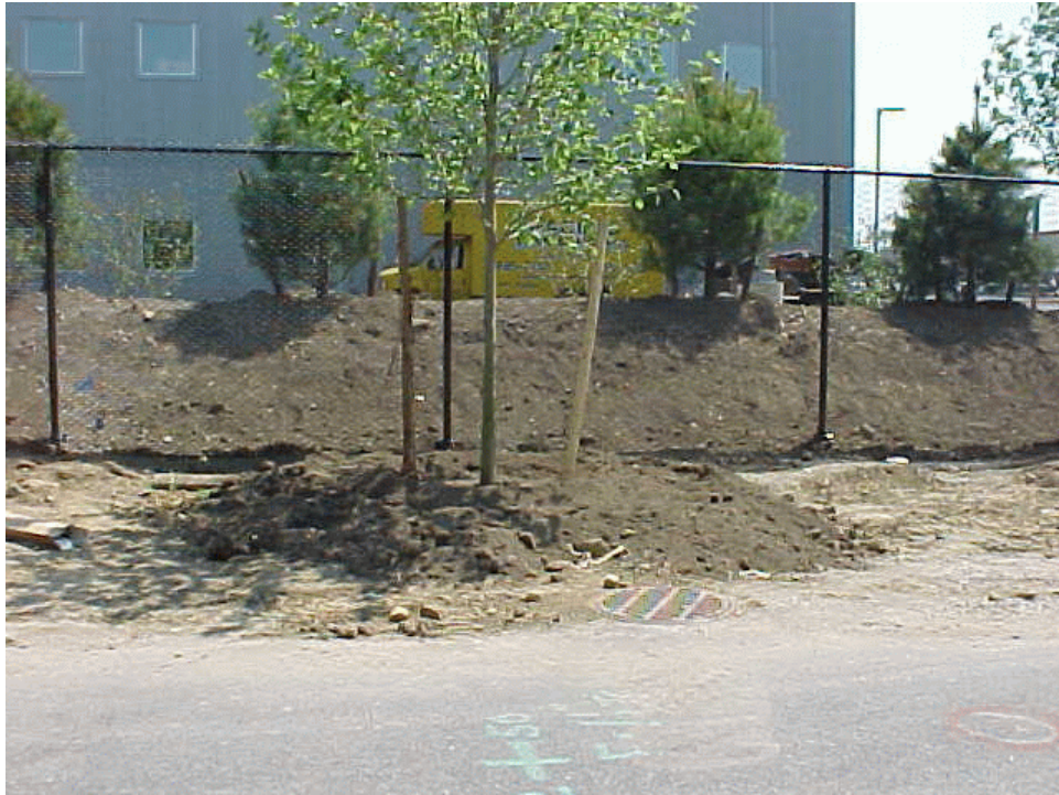
Photo 3: View south, from 15th Avenue, of second street inlet, site soil at inlet, and unstabilized soil in the background.
