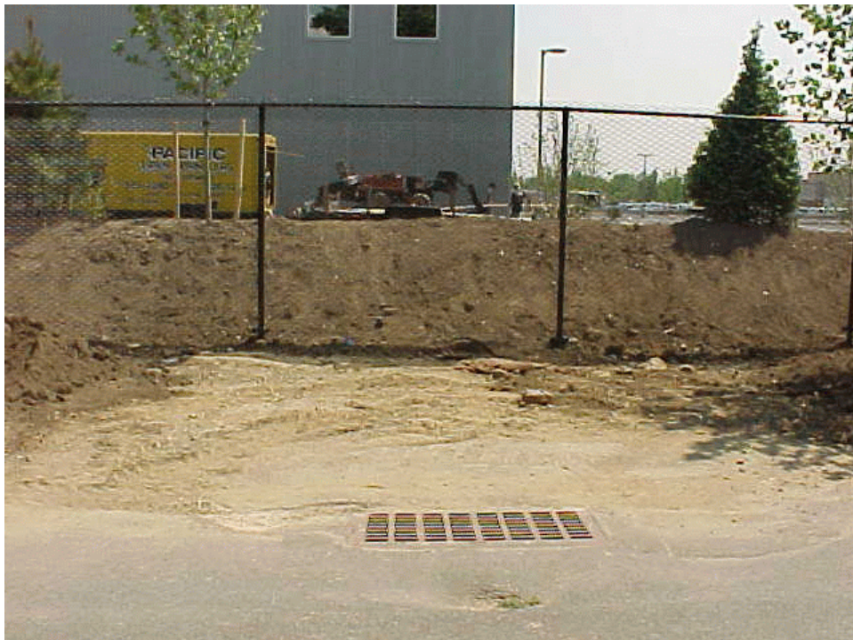
Photo 2: View south, from 15th Avenue, of a street inlet, site soil at the inlet, and unstabilized soil in the background.
