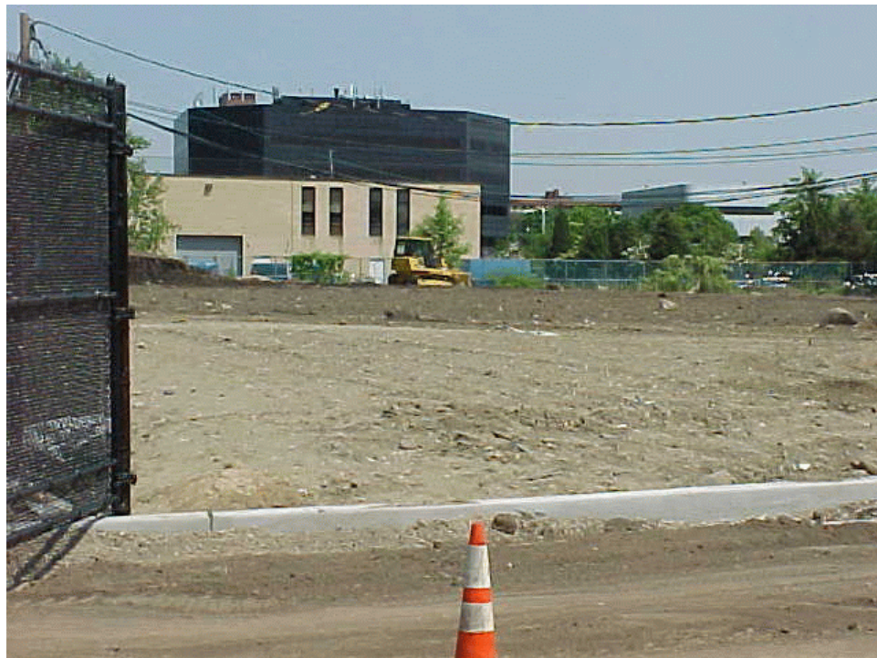
Photo 4: View southeast, from 15th Avenue, of bulldozer grading soil. Note the area had no visible BMPs.
