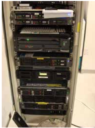
Fig 2. Legacy Data Center
