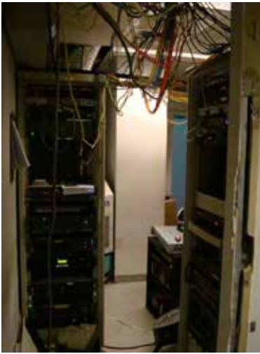
Fig 1. Legacy Data Center
