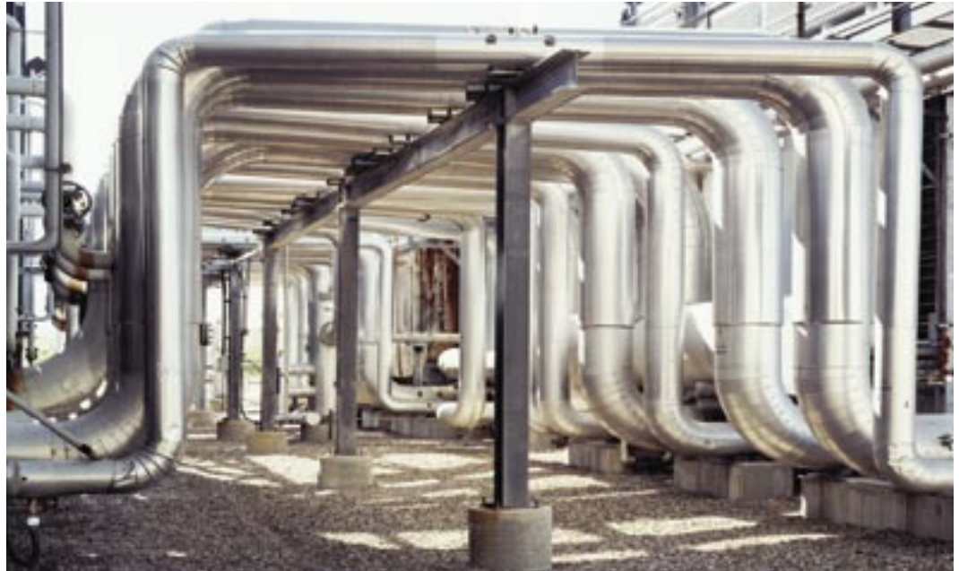
Before it can be injected into the ground, carbon dioxide is compressed, sent through these pipes to large cooling units, and compressed again.
