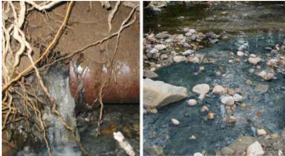
Figure 8 Raw sewage leaking from a broken pipe (left) into the Sligo Creek, which flows into the Anacostia (right). When a staff member of the Anacostia Watershed Society noticed raw sewage flowing in the creek, he notified Washington sanitation officials who claimed its source was a stormwater pipe under the jurisdiction of another agency. Continuing upstream, he found and photographed the real source of the sewage leak: a broken WSSC sewer pipe. 220 Photo source: Anacostia Watershed Society.
