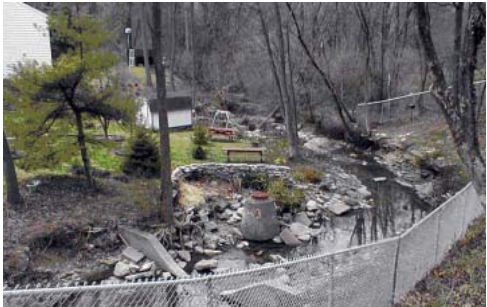
Figure 5 SSO 603 from which raw sewage spilled seven times in 2000 and nine times in 2001 into the E.B. Mill Creek, which flows through residential yards in Hamilton County, OH. 194
