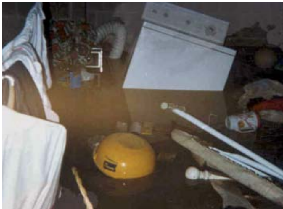
Figure 4 Basement Backup, Cincinnati, OH
