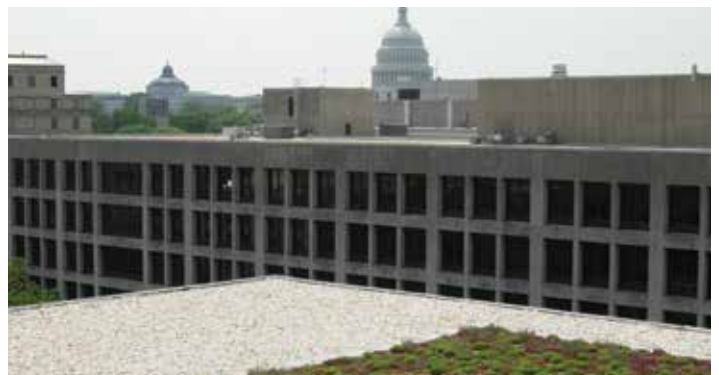
To help incentivize privately financed green roofs, Washington, D.C.'s Department of the Environment initiated a green roof subsidy program. The Department provides a rebate of $3 per square foot for installed green roofs; as a result, more than 50,000 square feet of green roof projects are under construction. The rebate has since grown to $5 per square foot.
